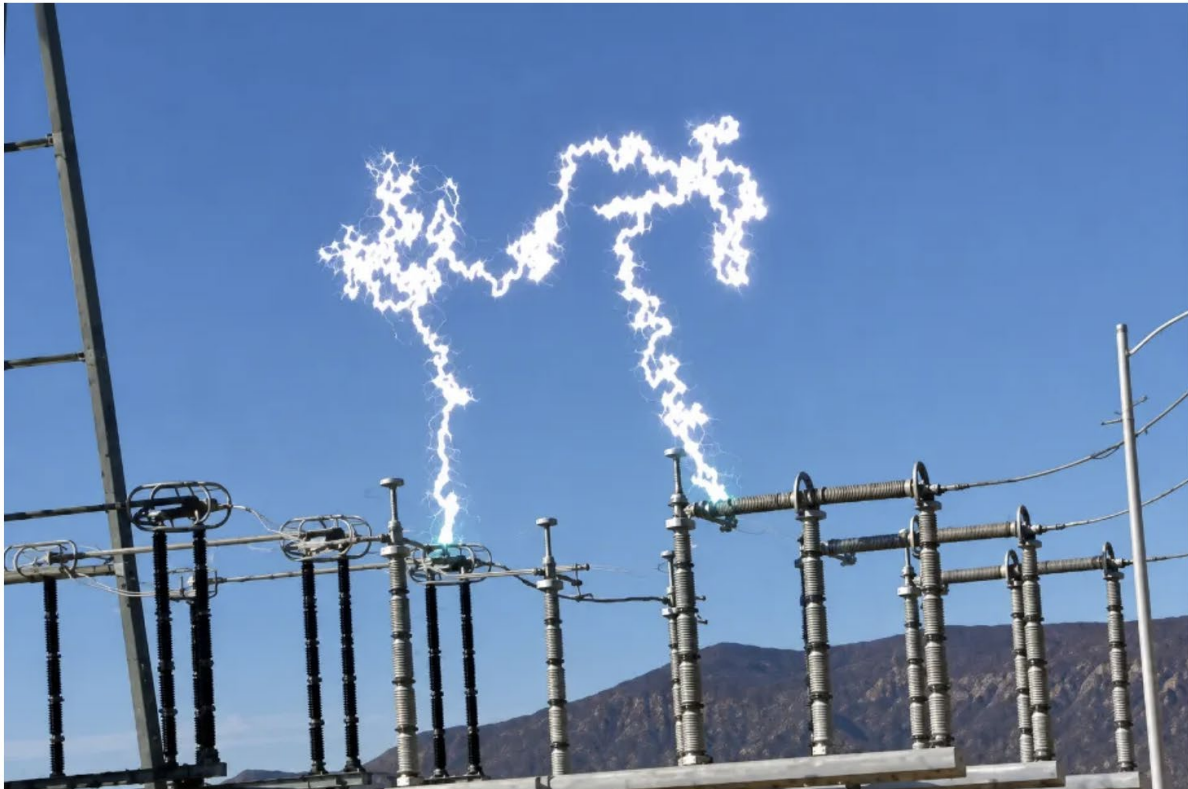
An electrical arc at a switchyard near Boulder City, Nevada. Credit: Capturedlightning.com
